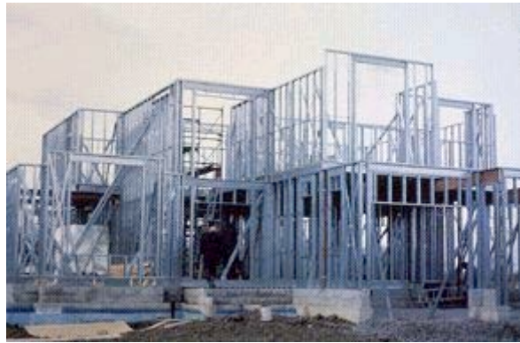
Source: Steel Framing Alliance
