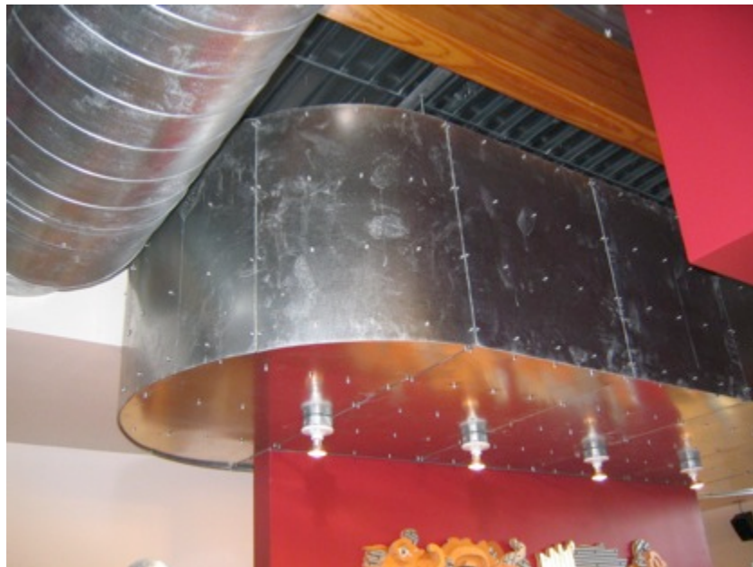
Figure 1 – Fingerprinting and handling marks on exposed galvanized ducting
