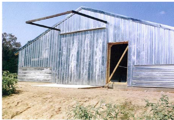
Building erected using roll-formed galvanized panels from a bundle that had extensive amounts of white rust.
