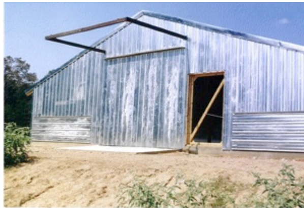
Building erected using roll-formed galvanized panels from a bundle that had extensive amounts of white rust.
