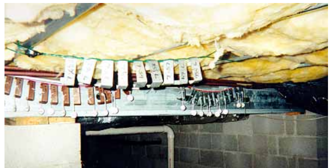
Figure 5 - Stud specimens in Leonardtown Site crawlspace. Note the uncoated C-sections in the background show red rust after just two months of exposure.
