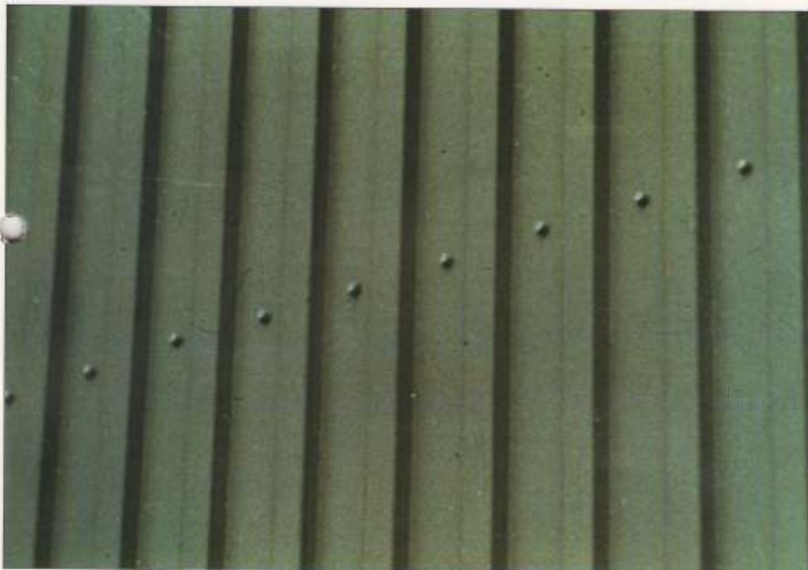
Fig. 10 Fixing holes on Ford Motor Company Depot — a potential danger point for corrosion, still in excellent condition after 10 years.
