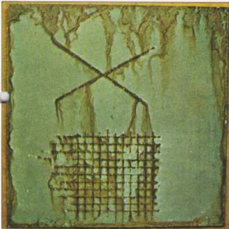
Fig. 2 Acrylic painted mild steel — Panel scribed through to steel substrate and salt spray tested to DEF 1053.
