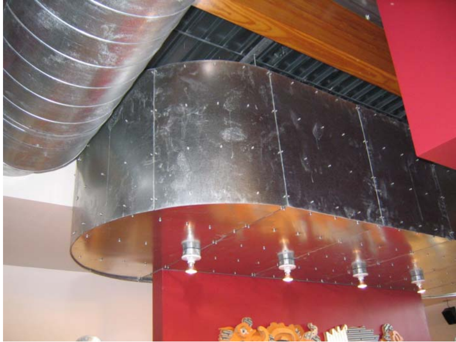
Figure 13 – Fingerprinting and handling marks on exposed galvanized ducting
