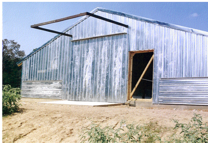
Figure 7 – Extensive storage stain (white rust) on sheets used to erect a storage building
